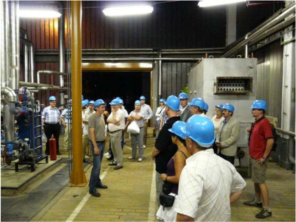
Participants in the boiler house of the Miskolc Heat Servicing Ltd. (MIHŐ Kft.) on Futó street, Miskolc, where the biogas boiler was installed
